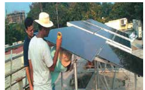
Outdoor testing of PV modules
