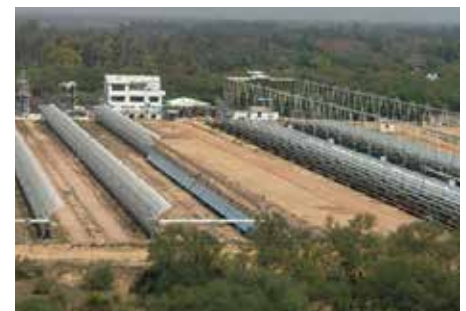
1 MWe solar thermal power plant
