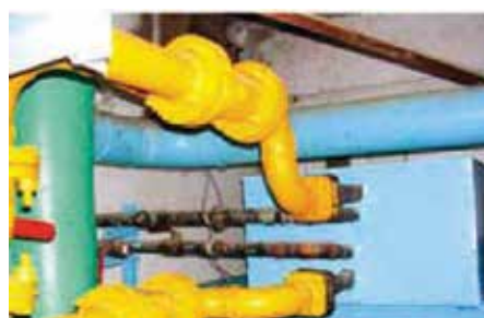
Tube-tube heat exchanger with piping
