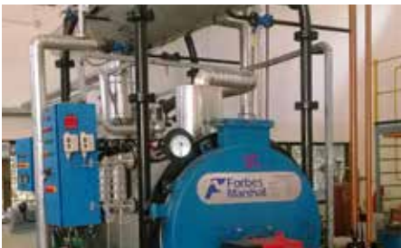
Forbes Marshall lab boiler
