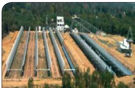
1MWe solar thermal power plant at Gurgaon
