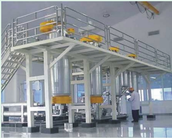
Supercritical Fluid Extraction Plant Designed at IIT Bombay
